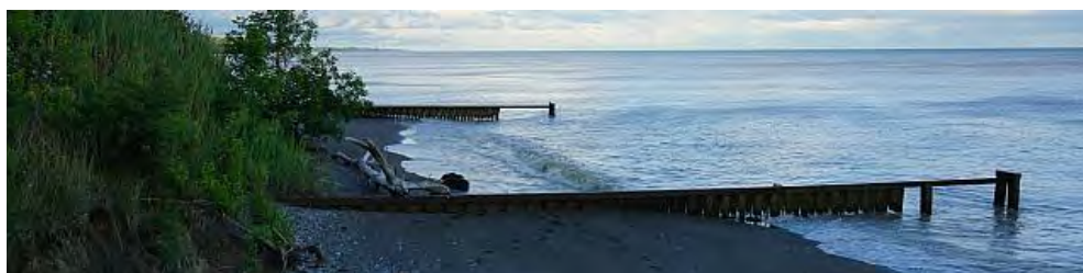
Figure 6.2 Steel Sheet Pile Groynes in Failure (top: sheet missing from the tip; bottom: vertical sheets corroded at the waterline)
