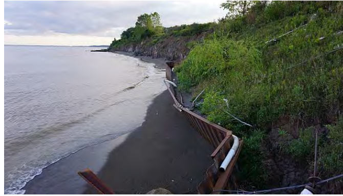
Figure 6.5 Failed Sheet Pile Wall due to Lack of Slope Design
