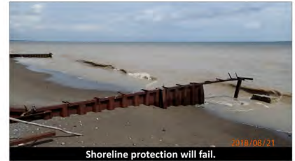
Shoreline protection will fail.
