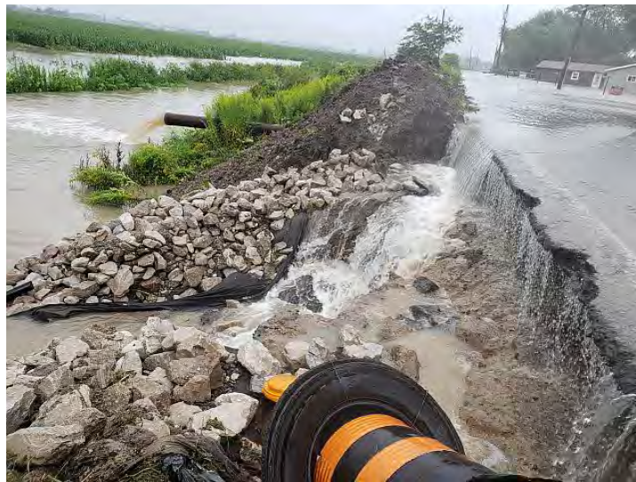
Figure 2.32 Erosion of Road Base, North Dike Slope and Flooding of Agricultural Fields, August 27, 2019 Storm
