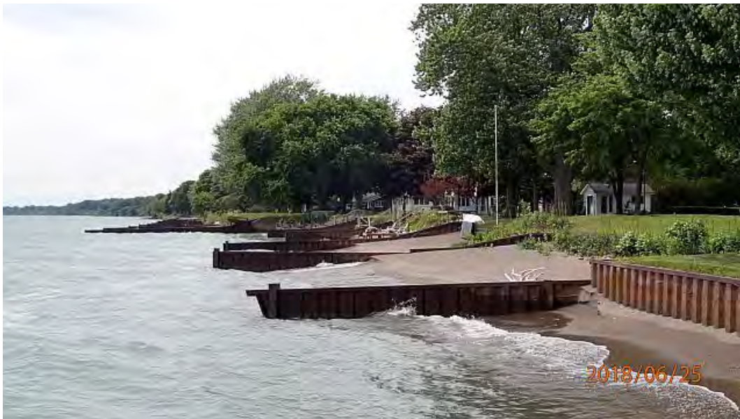
Figure 2.26 Steel Sheet Pile Groynes at Erie Beach
