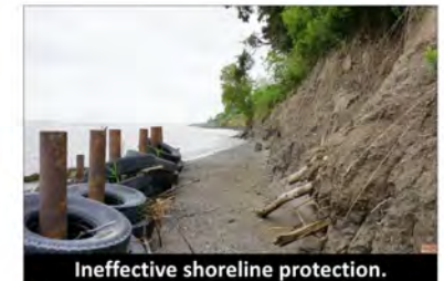
Ineffective shoreline protection.
