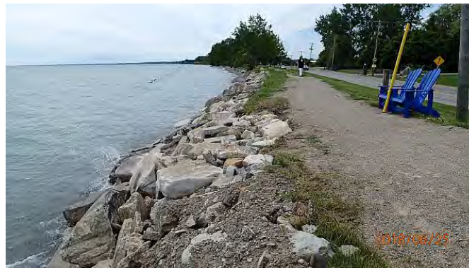
Figure 2.33 Armour Stone and Concrete Rubble in front of Dike, St. Anne’s Church
