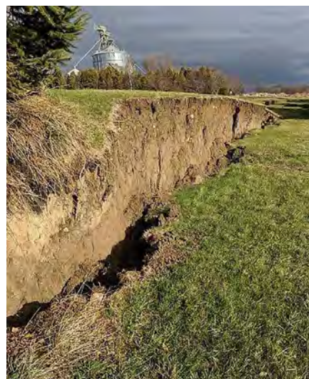
Figure 2.20 Port Alma Bluffs Tension Crack, November 2019
