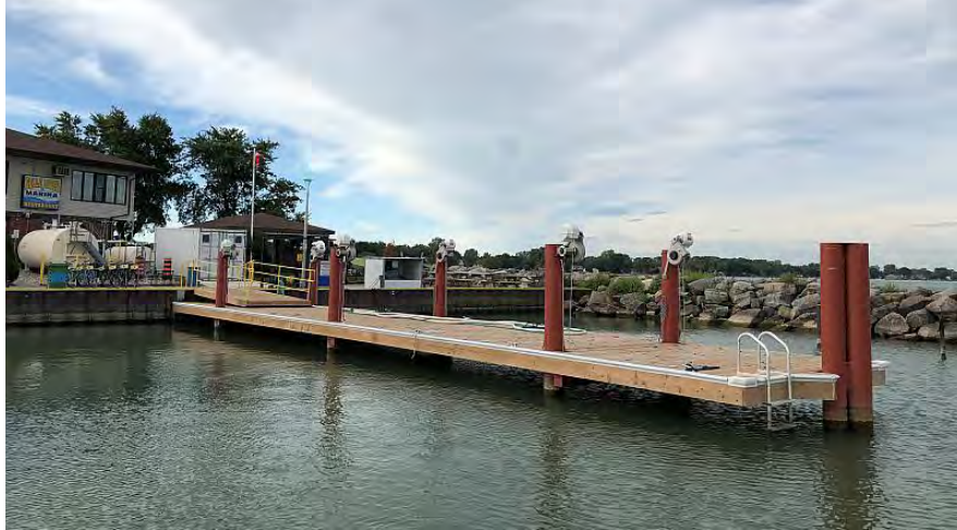
Figure 6.25 Adjustable Fuel Dock, Belle River Marina (2019)
