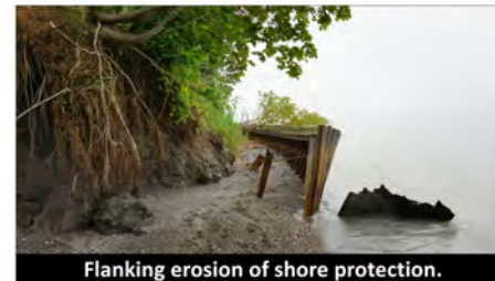
Flanking erosion of shore protection.
