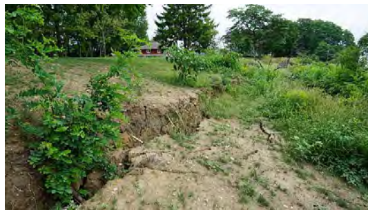
Figure 2.19 Formation of Tension Crack Along Bluff Crest
